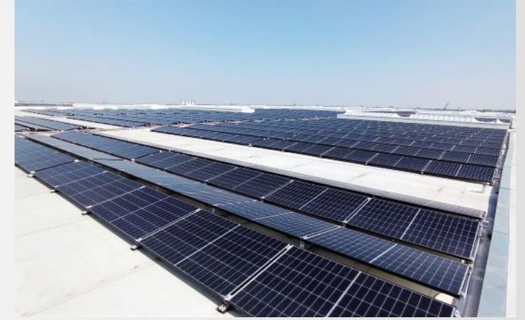
Castel San Giovanni (PC) 1300 kWp
