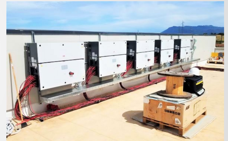
Colleferro (RM) 600 kWp
