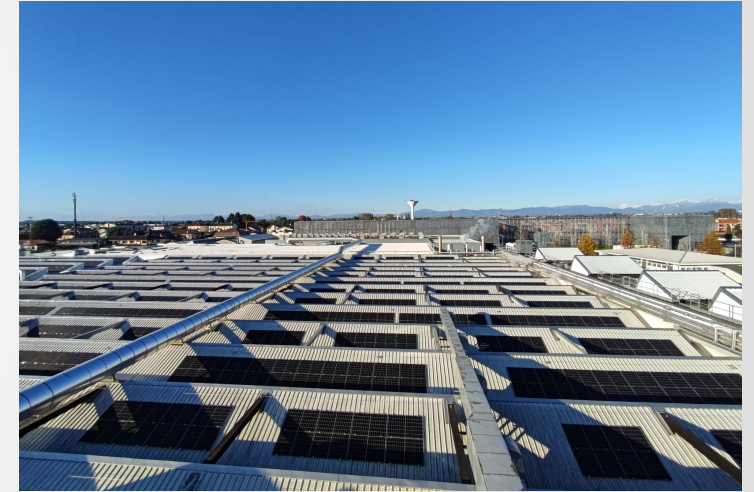
Lainate (MI) 1600 kWp
