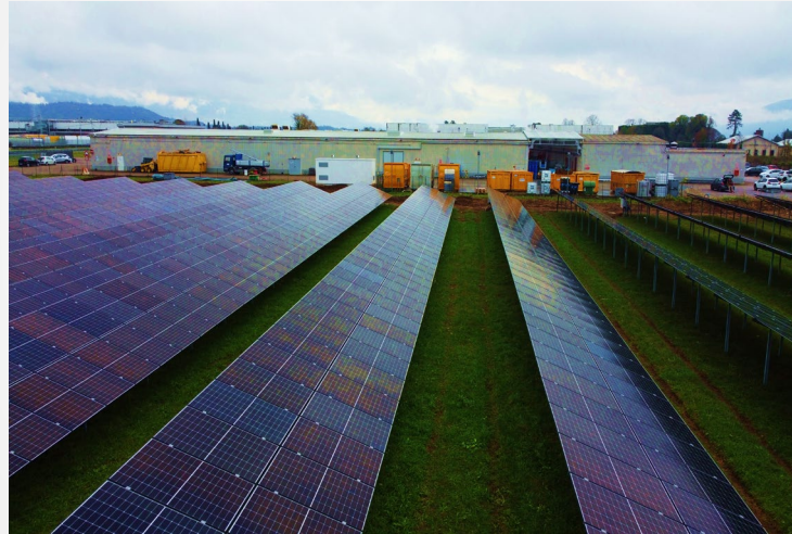
Gorizia (GO) 1000 kWp
