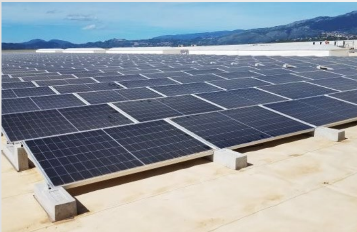
Colleferro (RM) 2000 kWp
