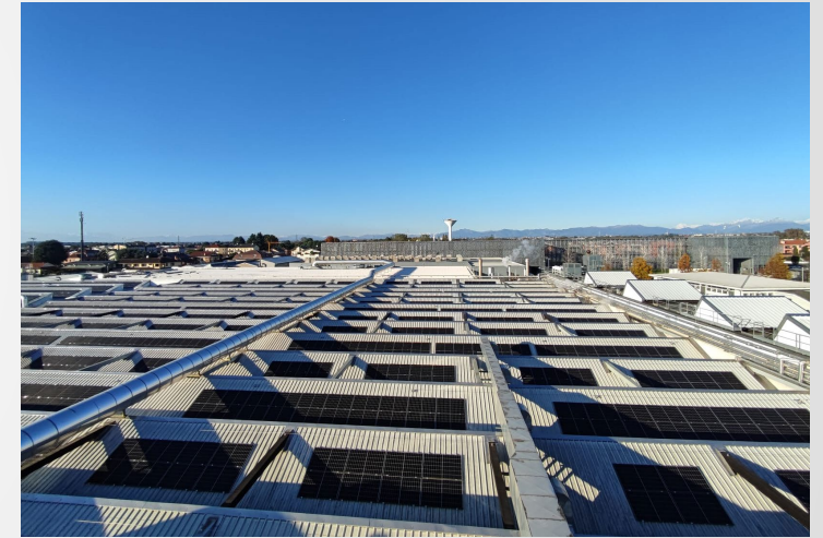
Lainate (MI) 1600 kWp
