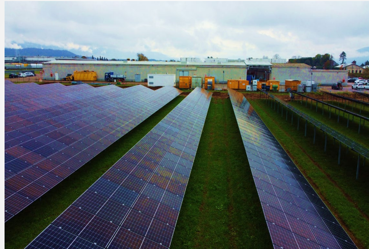
Gorizia (GO) 1000 kWp
