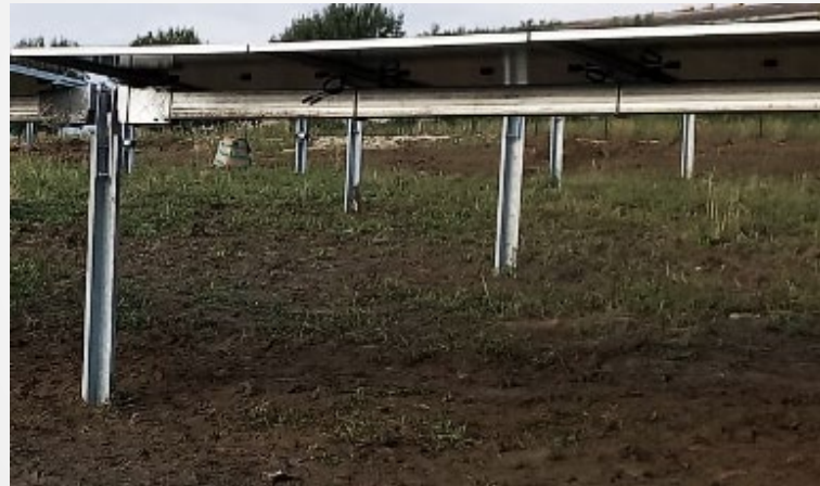
Castellana Sicula (PA) 1000 kWp Trackers
