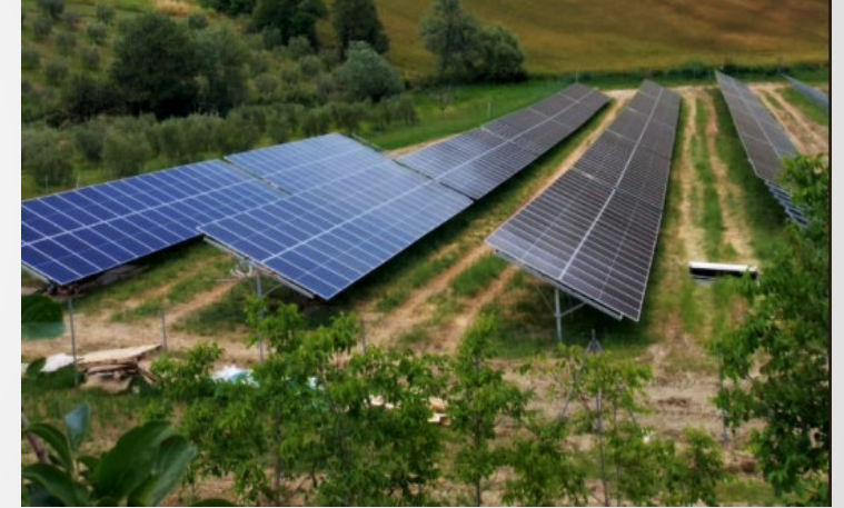
Barbara (AN) 811 kWp
