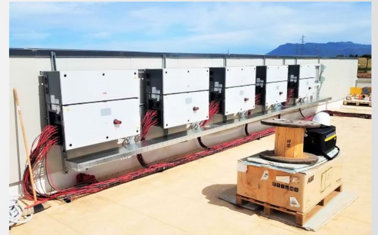
Colleferro (RM) 600 kWp
