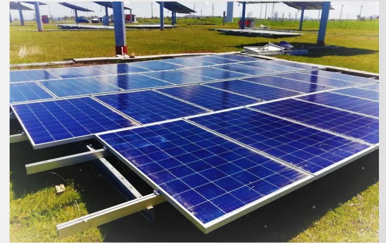
Vaglio Basilicata (PZ) 3000 kWp - trackers
