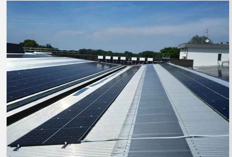
Parma (PR) 1000 kWp
