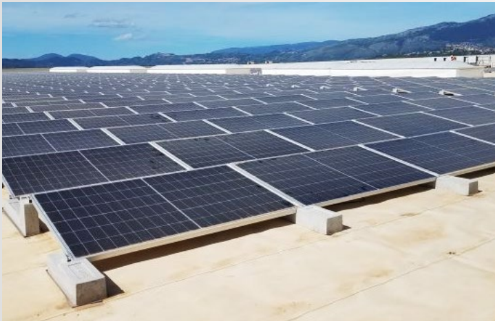
Colleferro (RM) 2000 kWp
