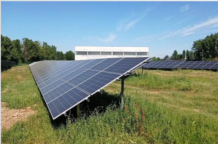
Capriano del Colle (BS) 880 kWp
